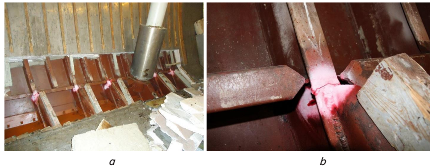
Fig. 2. Fatigue cracks in structural joints:
