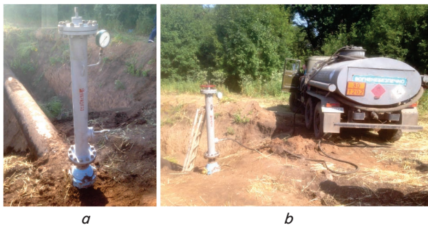
Fig. 2. Device for liquid removal from the pipeline ( a ) and the process of liquid drainage into a tank truck ( b )
