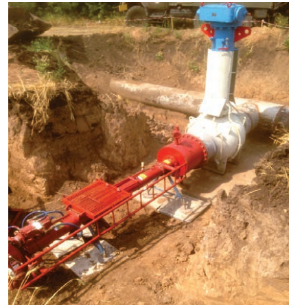
Fig. 3. TD Williamson hydraulically-operated tapping machine with the housing adapter mounted to the branch connection
