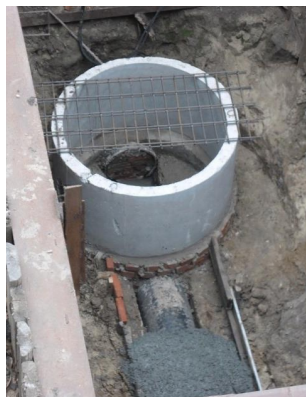
Fig. 5. Restoring conveyance capacity of the sewage header in Severin Pototsky Street: after the restoration works (RF5, Kharkiv, Ukraine, 2017)
