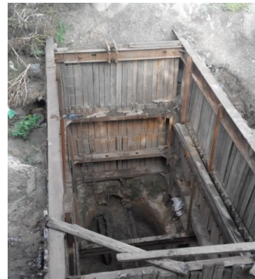
Fig. 4. Sewage header in Severin Pototsky Street before restoration (RF5, Kharkiv, Ukraine, 2017)
