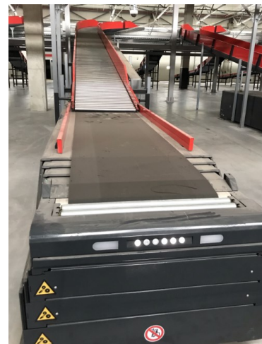
Fig. 8. Auxiliary lateral distribution conveyor of the logistics warehouse of Nova Poshta LLC in Soroky Lvivski village in Pustomyty district of Lviv region (Ukraine)
