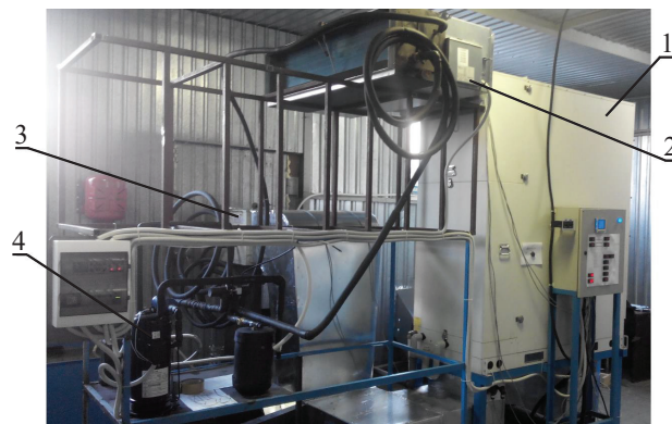
Fig. 2. Photograph of the installation of air heat supply according to the combined thermodynamic cycle with heat recuperation: 1 – the M-cycle heat-and-mass exchanger; 2 – the heat pump condenser; 3 – the heat pump evaporator; 4 – the heat pump compressor
