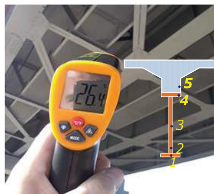
Fig. 2. Temperature measurement at the surface of the reinforced concrete beam of the bridge
