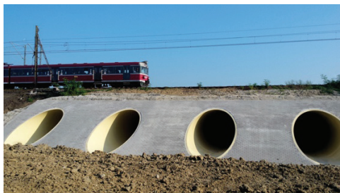
Fig. 1. The operation process of fiberglass pipes in the body of a railroad embankment [1]
