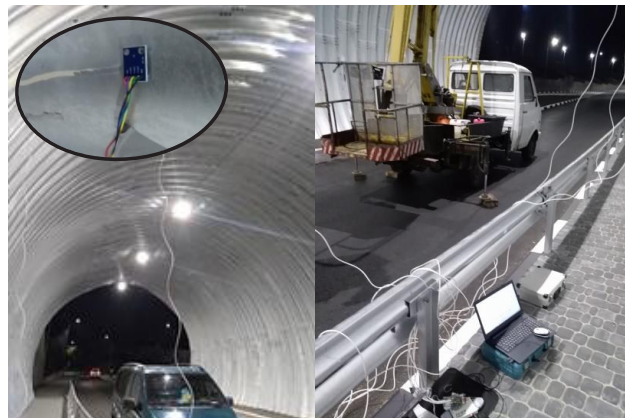
Fig. 4. Inertial experimental tests of the tunnel overpass made from prefabricated metal corrugated structures
