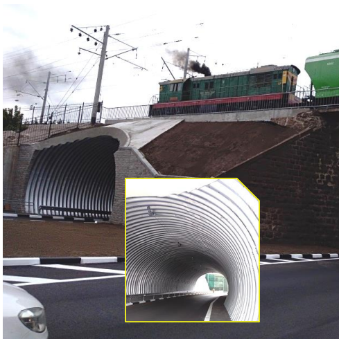
Fig. 1. General view of the tunnel overpass made from prefabricated metal corrugated structures under a railroad track
