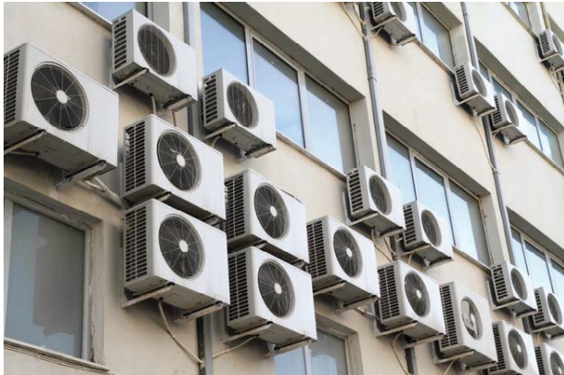
Fig. 2. An example of improper installation of external air conditioner units on the façade of the building
