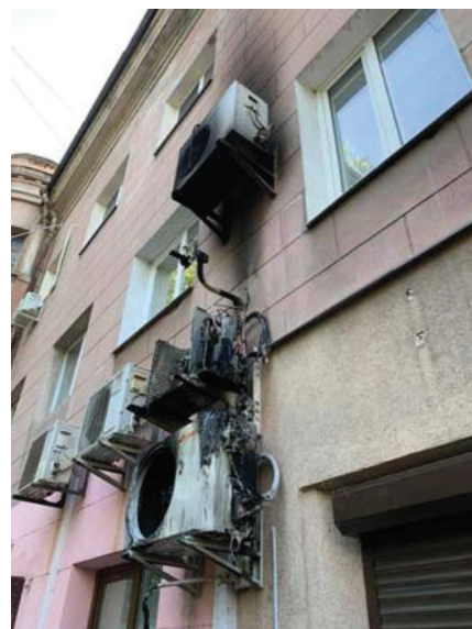
Fig. 1. Photograph of the consequences of the fire in the vertical arrangement of air conditioners
