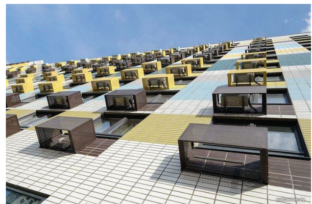
Fig. 3. An example of a façade system equipped with baskets for external air conditioner units with a decorative aluminum composite panel
