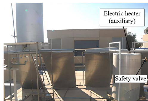
Fig. 3. Second storage tank containing a heater
