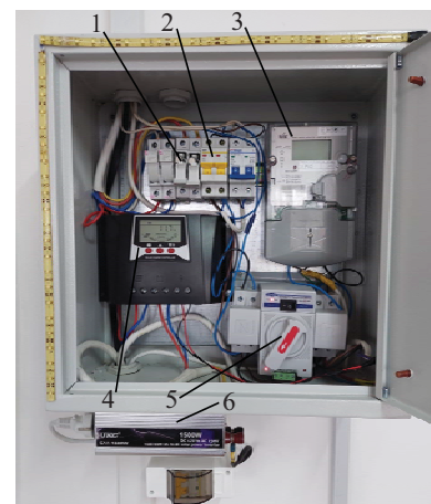
Fig. 6. Control system cabinet: 1 – fuse switch of solar panels (25 A); 2 – circuit breaker-automate of centralized lighting system 220 V (15 A); 3 – electricity meter NIK 2104 (single phase, RS-485); 4 – charge-discharge controller WP8048 PWM (80A, 12V/24V/48V); 5 – device for automatic activation of reserve TOMZN (single phase); 6 – inverter UKC SAA-1500W (DC 12V-AC 230V)
