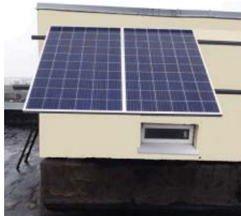
Fig. 4. Solar panels Photovoltaic JKM280PP-60-V, installed on the roof of the educational building
