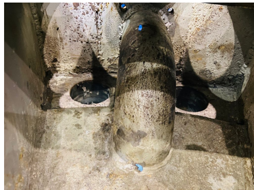
Fig. 6. Elbow inside the balance pipe of the head cover [23]
