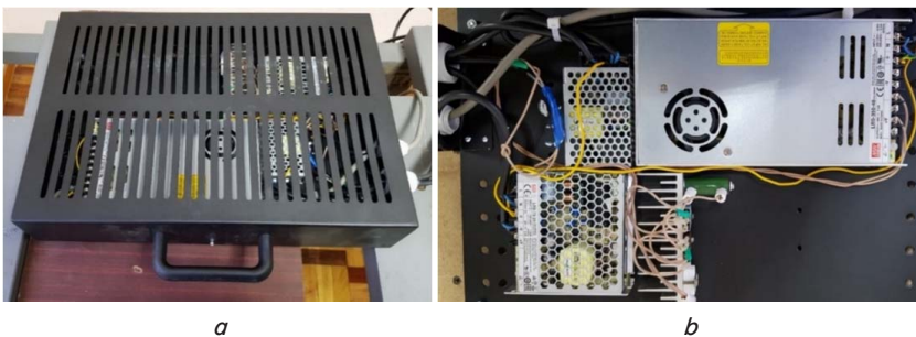
Fig. 5. Power supply equipment of the supporting and rotating device: a – general view of the power supply unit; b – placement of modules in the power supply unit
