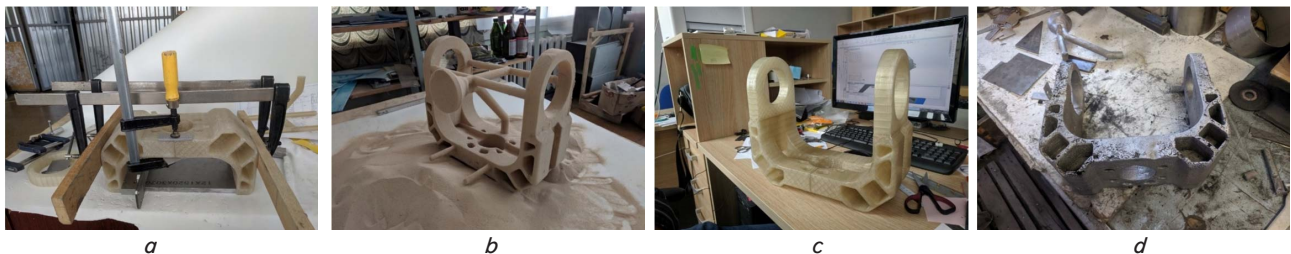
Fig. 1. Production of a supporting frame for the supporting and rotating device: a–c – the process of building a mold for casting the frame; d – cast frame before processing
