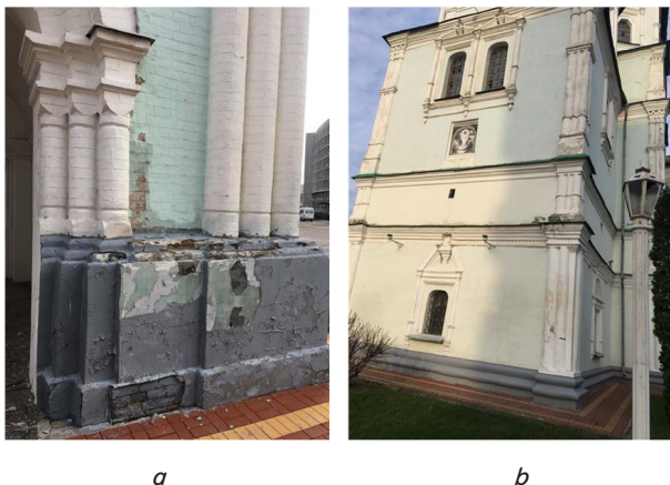
Fig. 1. Image of external damage to the facade of the Holy Resurrection Cathedral:
