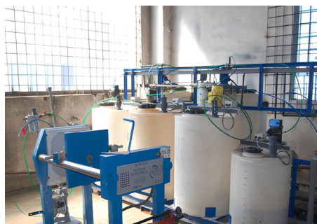
Fig. 2. Wastewater treatment facilities at the “Hardware Products Factory” LLC
