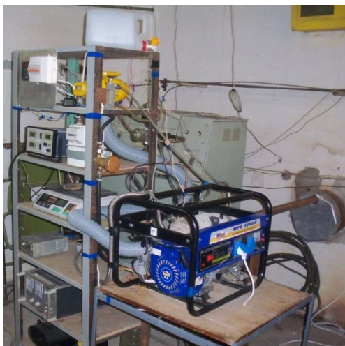
Fig. 1. General view of a power plant with a thermochemical conversion reactor
