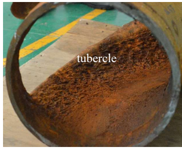
Fig. 1. Erosion corrosion condition on the inner surface of the pipe
