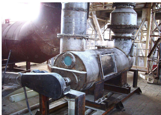
Fig. 2. Image of the pilot experimental installation for studying the process of hydrogen sulfide desorption in HDBD
