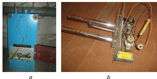
Fig. 6. Image of an automatic gas burner in a fuel boiler: a – fuel boiler; b – automatic gas burner with temperature control
