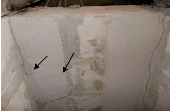
Fig. 8. Peeling of CLP series plaster during the curing of the structure
