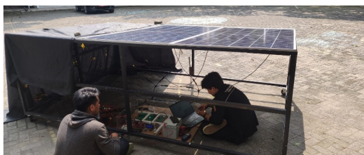
Fig. 9. MPPT system testing
