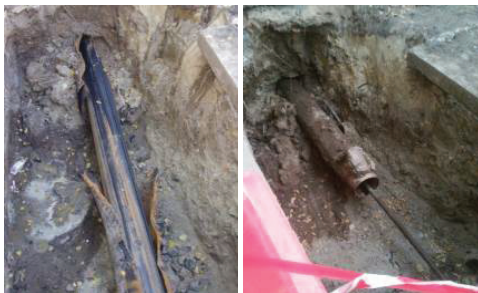
Fig. 10. «Extrusion» of the existing pipe from the ground massif at OR1 in Prospect Nauky Avenue (September 2015)
