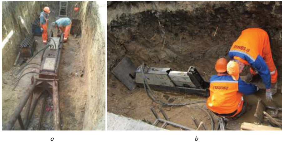
Fig. 8. Technological operations of the «Berstlining» method: a – installation of equipment into the target trench in Prospekt Nauky Avenue (September 2015), b – pushing the steel rods inside the worn pipeline in Trinkler Street (June 2016)
