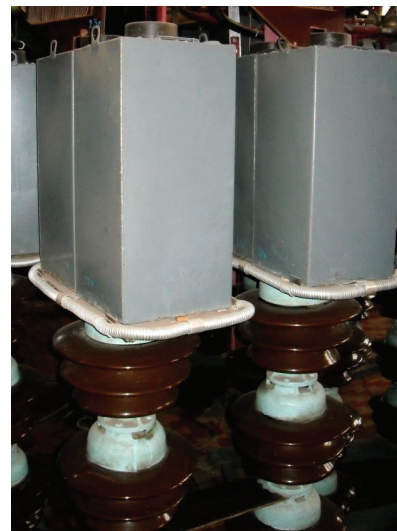
Fig. 4. Installation of IC-50-3 capacitors on support insulators to provide the necessary insulation from the ground in the impulse voltage generator
