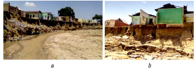
Fig. 8. Washing, scouring and undercutting of sandstones around houses at: a – site A; b – site C axis
