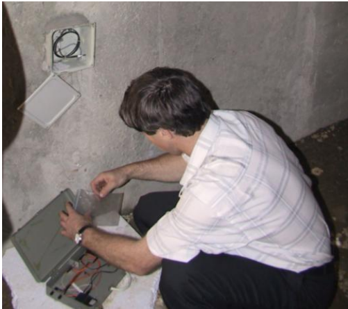
Fig.5. Voltage control in a reinforced concrete pylon of the basement of a multi-storey building
